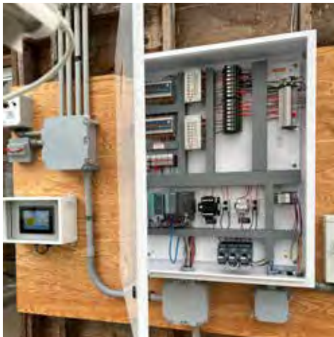
The Seed system stores data inputs and outputs and uses smart technology to control the greenhouse environment. A touchscreen control box (left) allows for monitoring and control of the Seed system.
