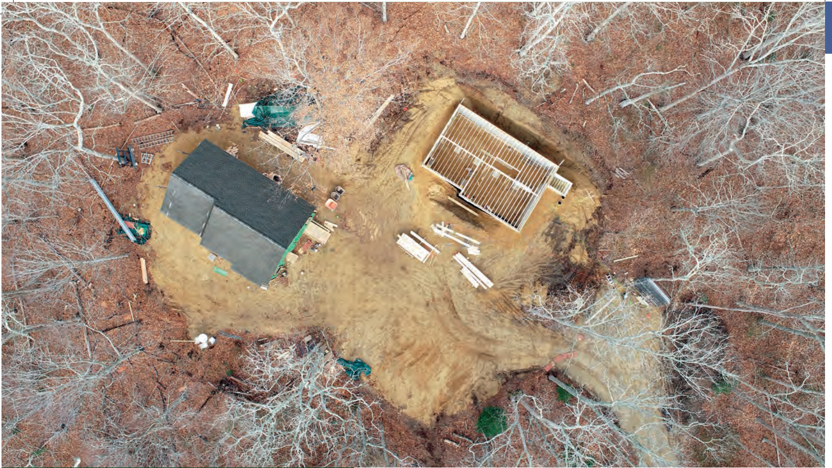
An aerial view of the two staff housing units under construction just north of our Visitor Center
