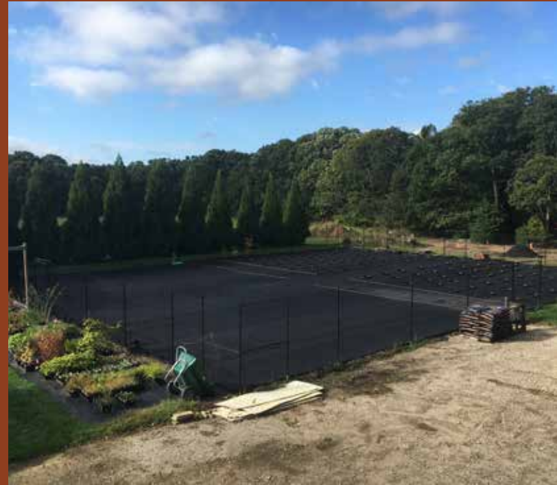
2018: The recently installed nursery is ready to accept trees growing in the greenhouse. Note how the Yoshino Japanese cryptomeria have grown into an effective windbreak.
